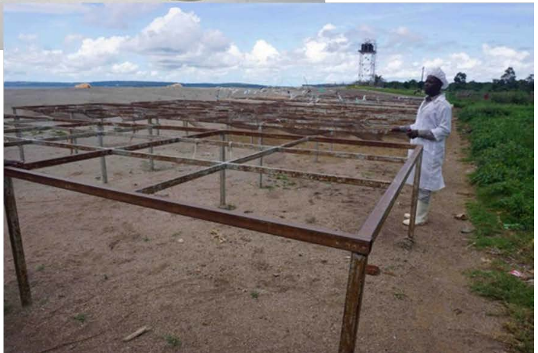
Kasekulo-Ttubi Fish Landing Site. Water supply house with solar power. Broken tap in the yard. Two chambers for filling in chlorine for disinfection, and chemicals available on site (used every day). The operator had seemingly good knowledge of the operation. The fish drying rack in Kasekulo-Ttubi village not in use – rusty and broken.
