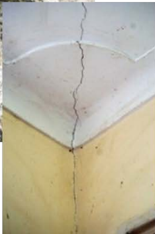
Mazinga Sub-County Office in standard design. Showing some signs of deterioration, e.g. hole in water tank (not in use) and rotten latrine doors. The ceiling in the assembly hall has a large crack. The building exterior needs brush-up painting.
