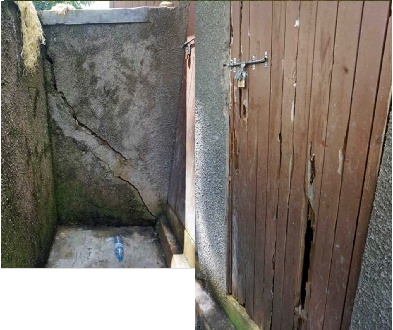
Bufumira Sub-County Office. (No-one at home when visiting, but doors were open). Nice main building with solid furniture, but deteriorating latrine structures, with broken plastering and termite-eaten/rotten latrine doors of wood.
